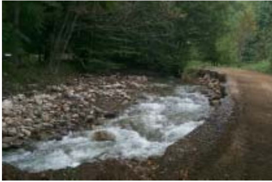
Creek bank damage after storms.
