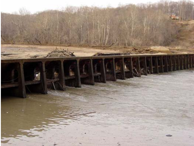
Ten sections breached in Embrey Dam on the Rappahannock River, Virginia.
